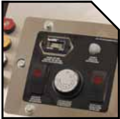
Control panel includes 120V/15-amp auxiliary switch for a duplex GFCI outlet*
